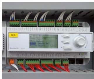
Controller box upgrade
